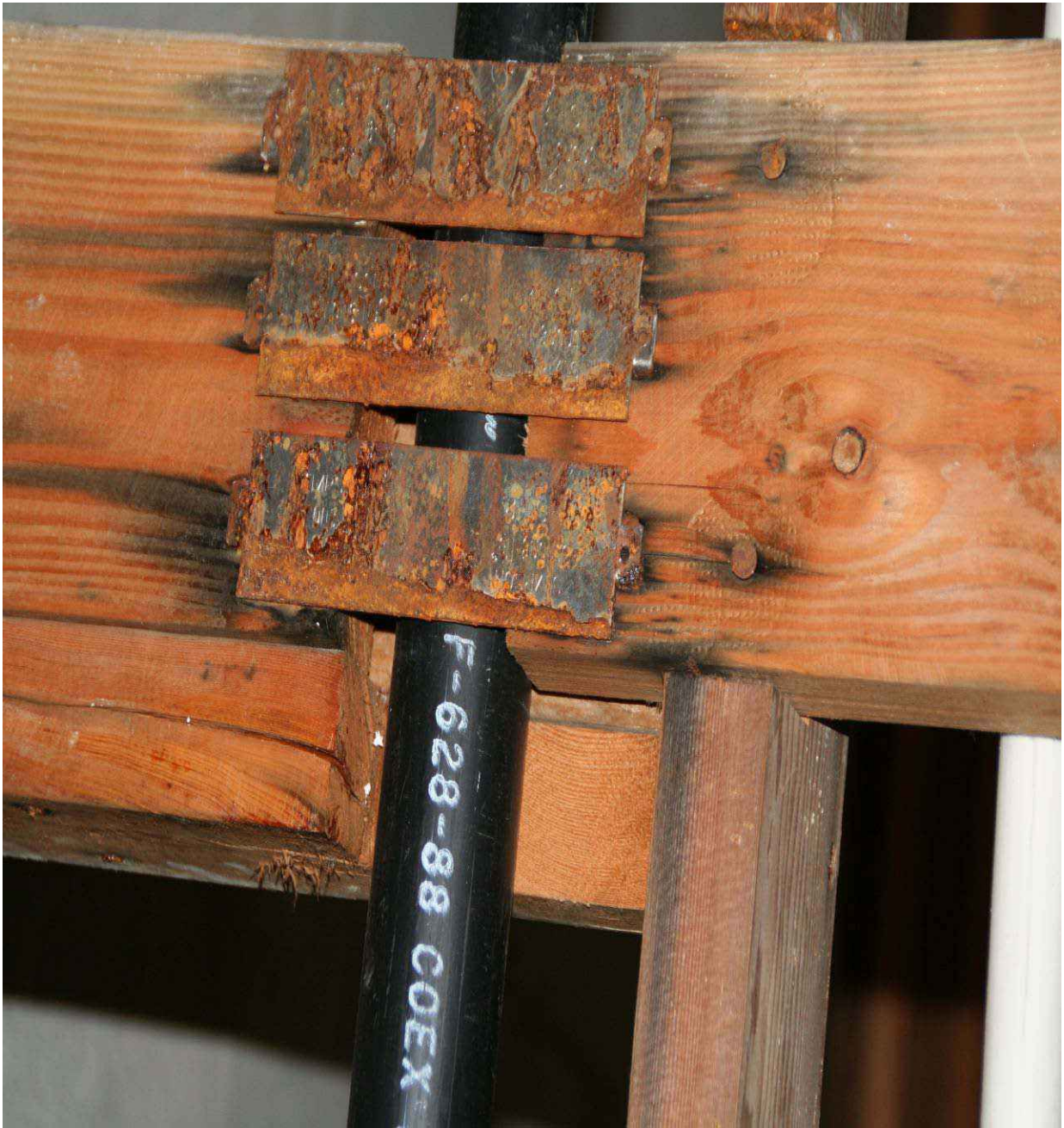
Building framing with wood staining from metal clips (staples).
