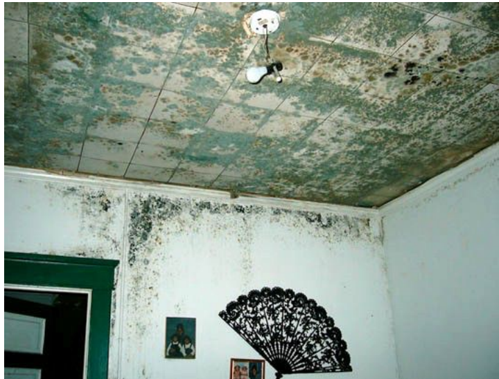
Mold growing on the ceiling and walls of a house after Hurricane Katrina
