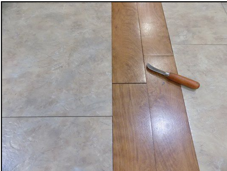
Gaps from tile shrinking over a hot substrate
